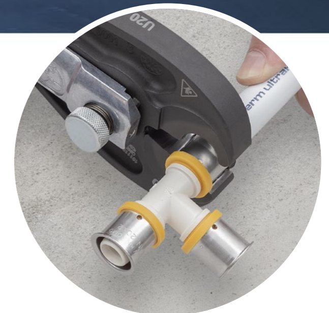
06 | Unlocking and removing the jaw from the fitting. The connection is ready for a leak test.
